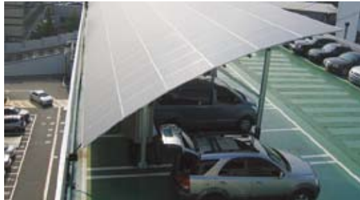
* Solar power generator system at the Suwon Service Center
